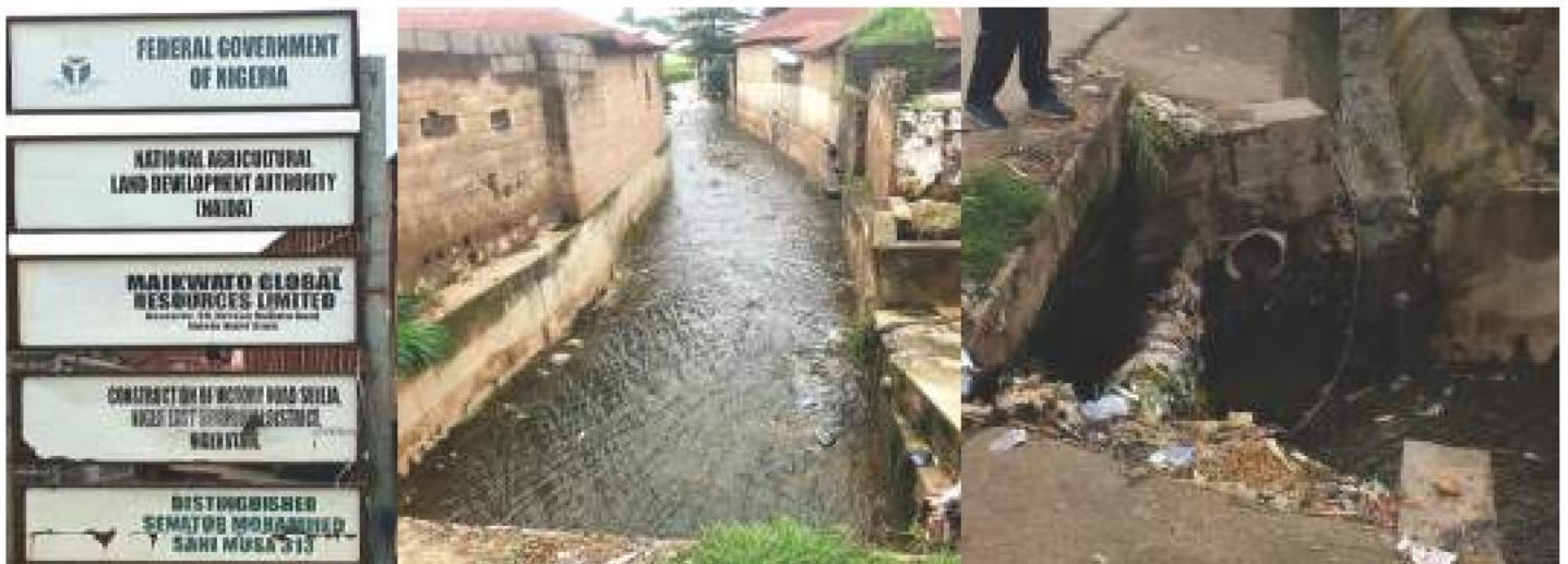
Figure 5: Pictures of Ecological Fund-supported Gully Erosion Control Construction Works Project at Bida, Niger State.
