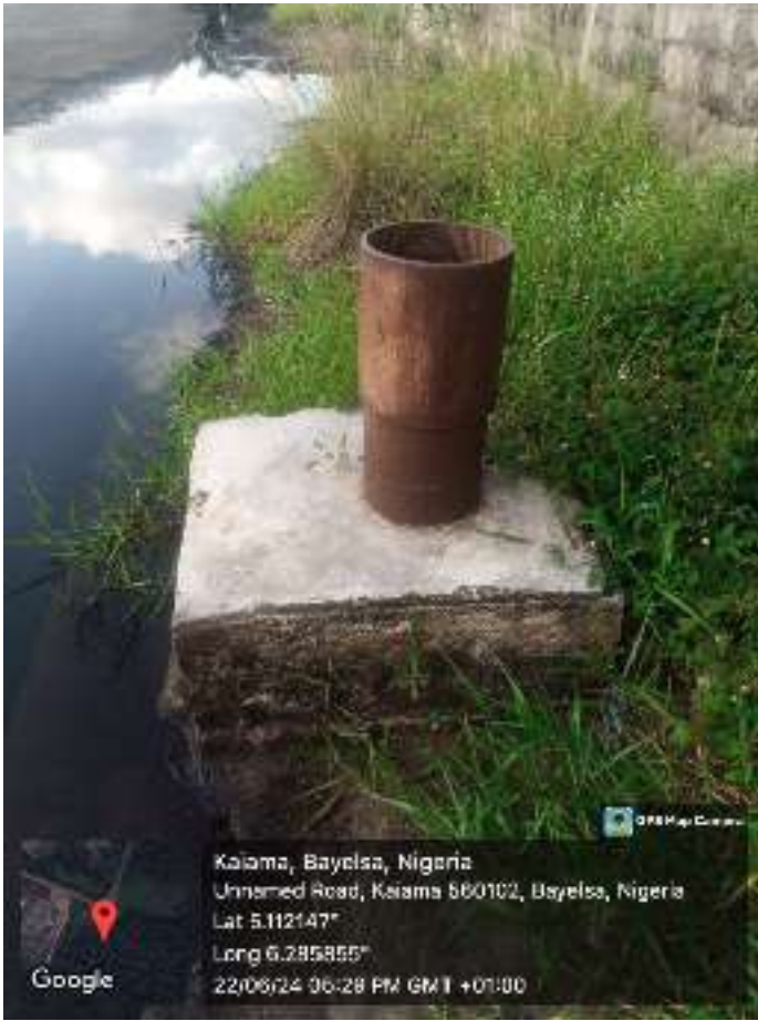
⬇️ Picture showing land erosion in Brass Local Government
